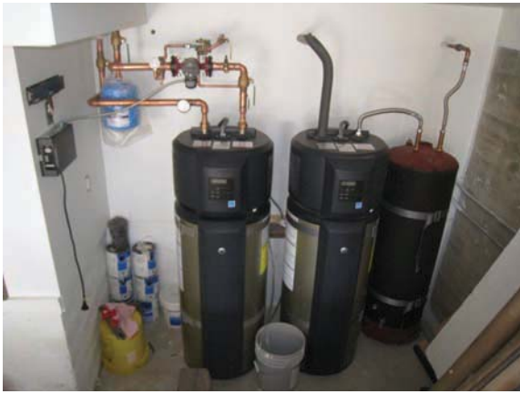
Water tanks in the passively heated garage
