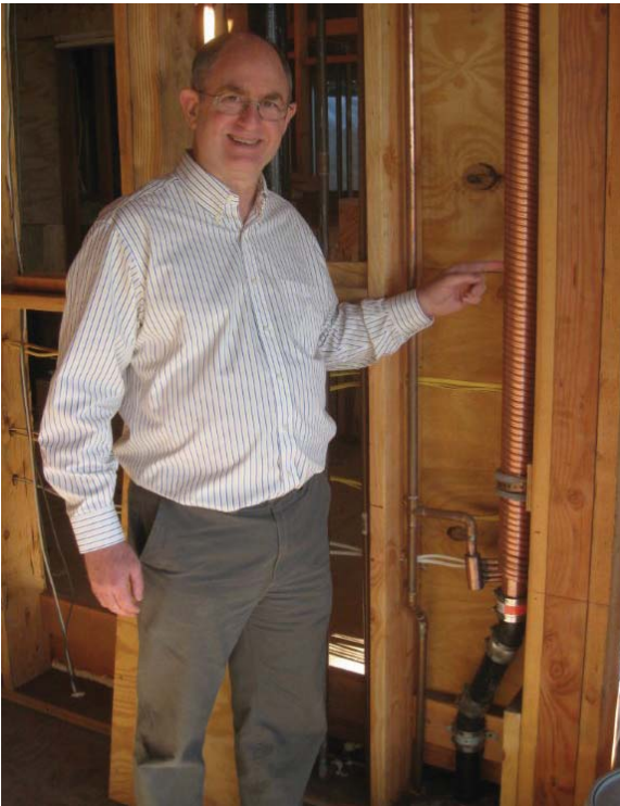
Hot water expert Gary Klein shows the upstairs Power Pipe Drain Water Heat Recovery Unit.
